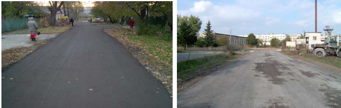
Fig. 3 General view of surface course from cold mixes based on milled asphalt concrete after compaction (left image – composite binder, right image – cement)
